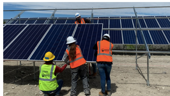
NortonLifeLock partners with GRID Alternatives to bring solar energy to underserved communities.
